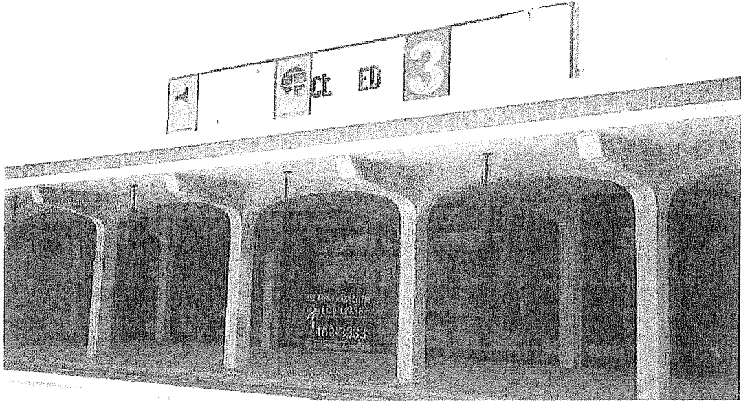
Figure 6A: One of two vacant movie theaters at Town & Country Mall that face the Sam Houston Tollway.
