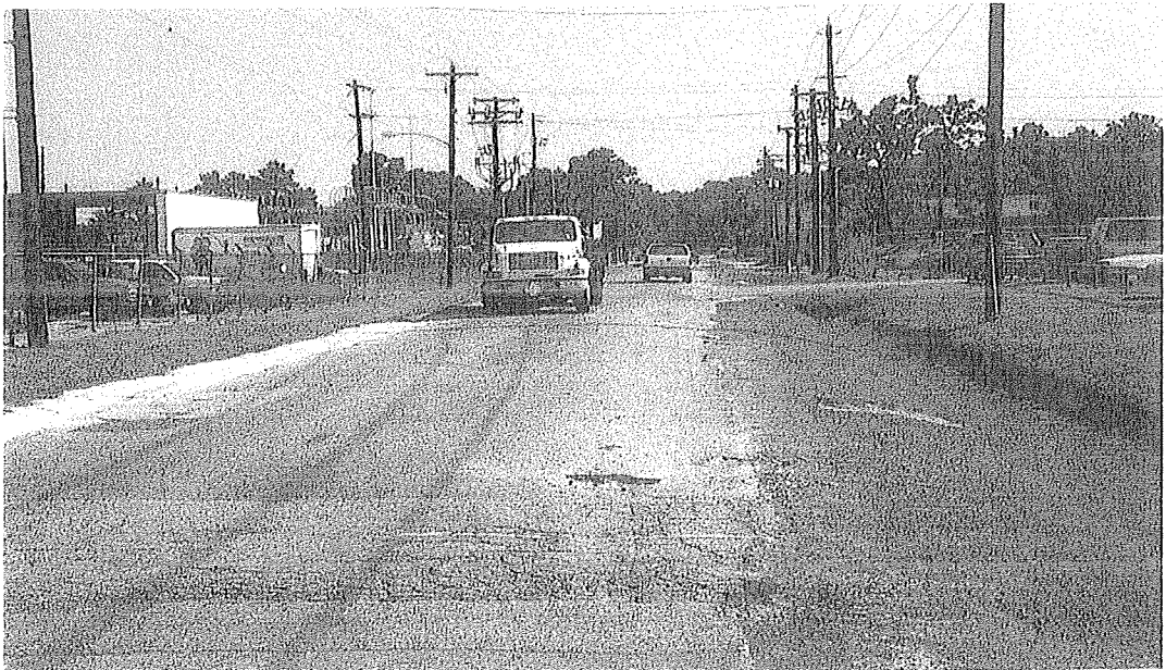
Figure 8: North side commercial area roadway without adequate drainage, sidewalks, or capacity.
